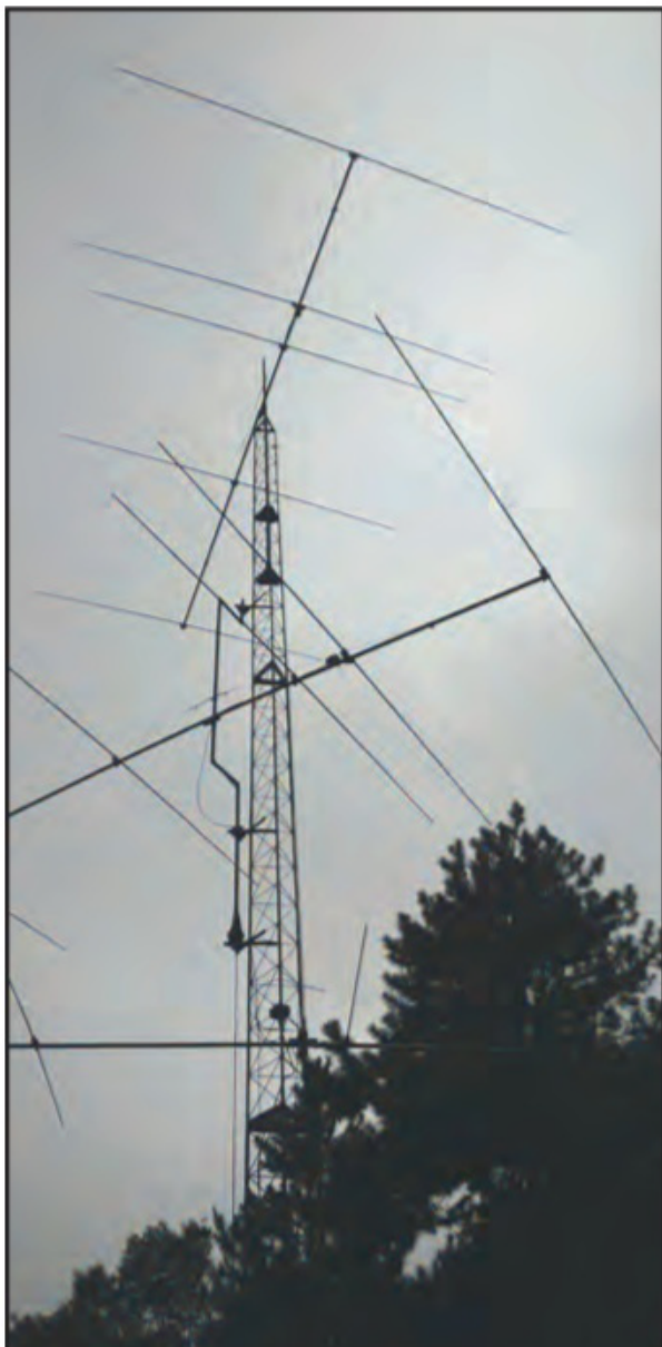
15-meter stack at PX2A.
