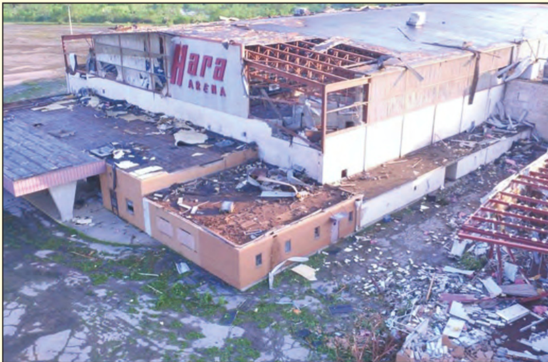
This drone image shows just some of the damage inflicted on Hara Arena, former home of the Dayton Hamvention®, by an EF-3 tornado on May 27. The complete drone video of the scene is online at < https://tinyurl.com/y3d4u5lt >. (WHIO-TV photo)
